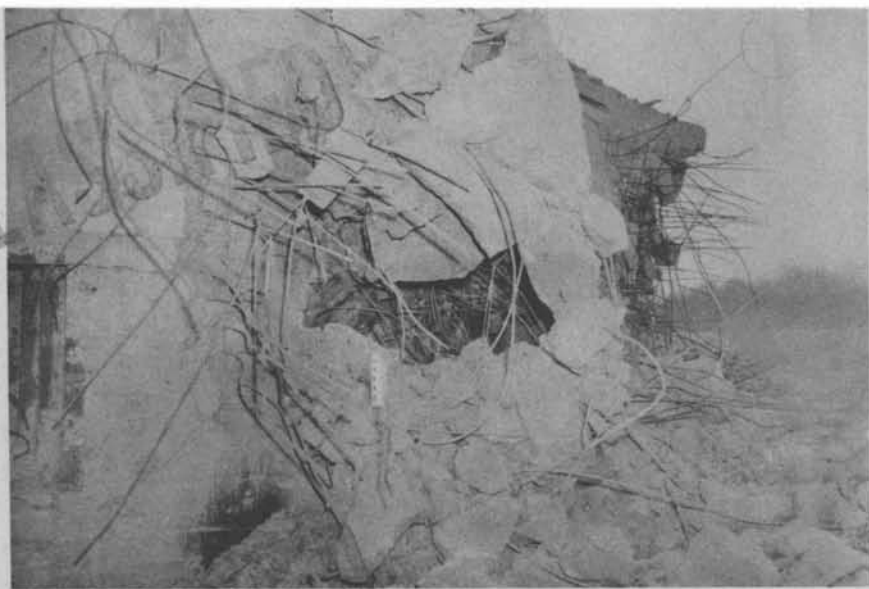
Gun, 155 mm, M1A1 firing Shell, H.E., 155 mm, M101 with Fuze, CP, M78. Range 2,400 yd. using supercharge. Crater 84 in. deep, 148 cu. ft. of reinforced concrete removed. Wall completely perforated. This is an exceptional round, results consistent with this can not be expected with all rounds fired, as results at this range gave less penetration.
